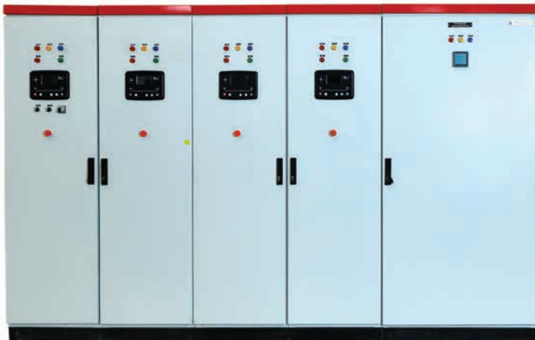
4 GENSET SYNCHRONIZING PANEL
