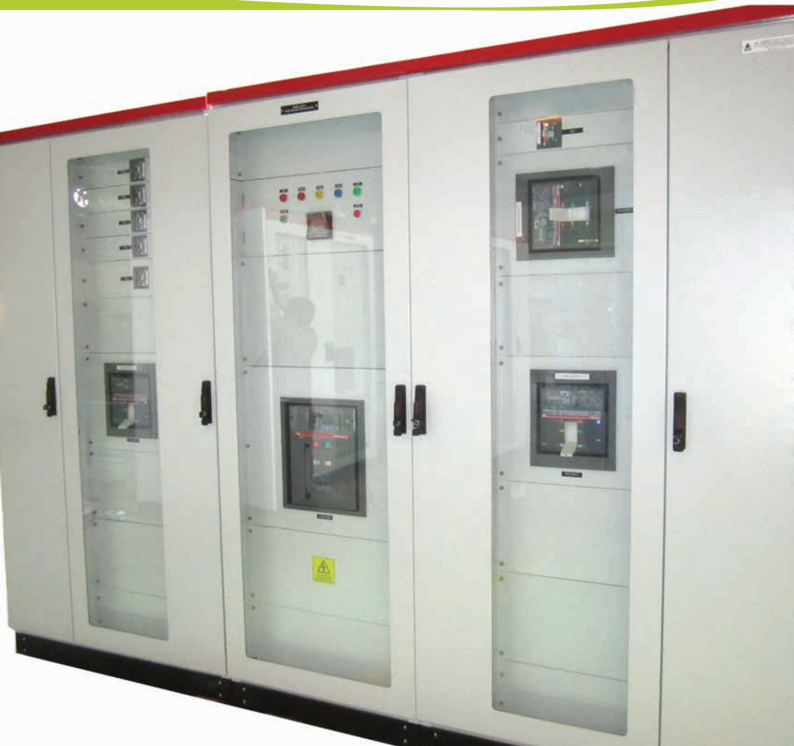
2500A MAIN DISTRIBUTION PANEL
